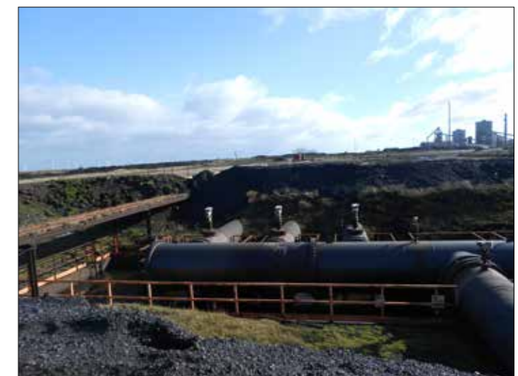
RBT - Estuary water mains - Valve chamber
