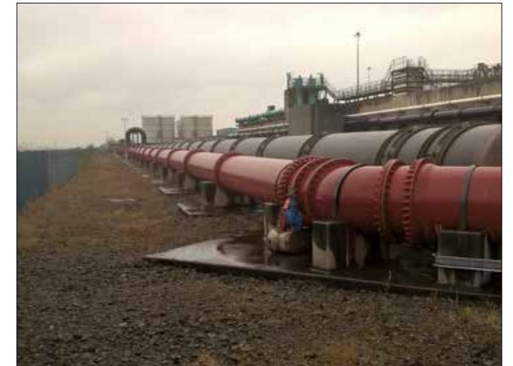
WWTW Sewage Transfer Mains
