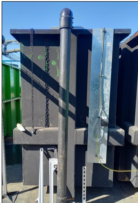
Figure 12. Backwash tank T4
