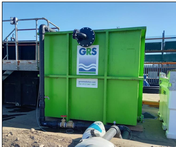
Figure 7. Inlet tank T1
