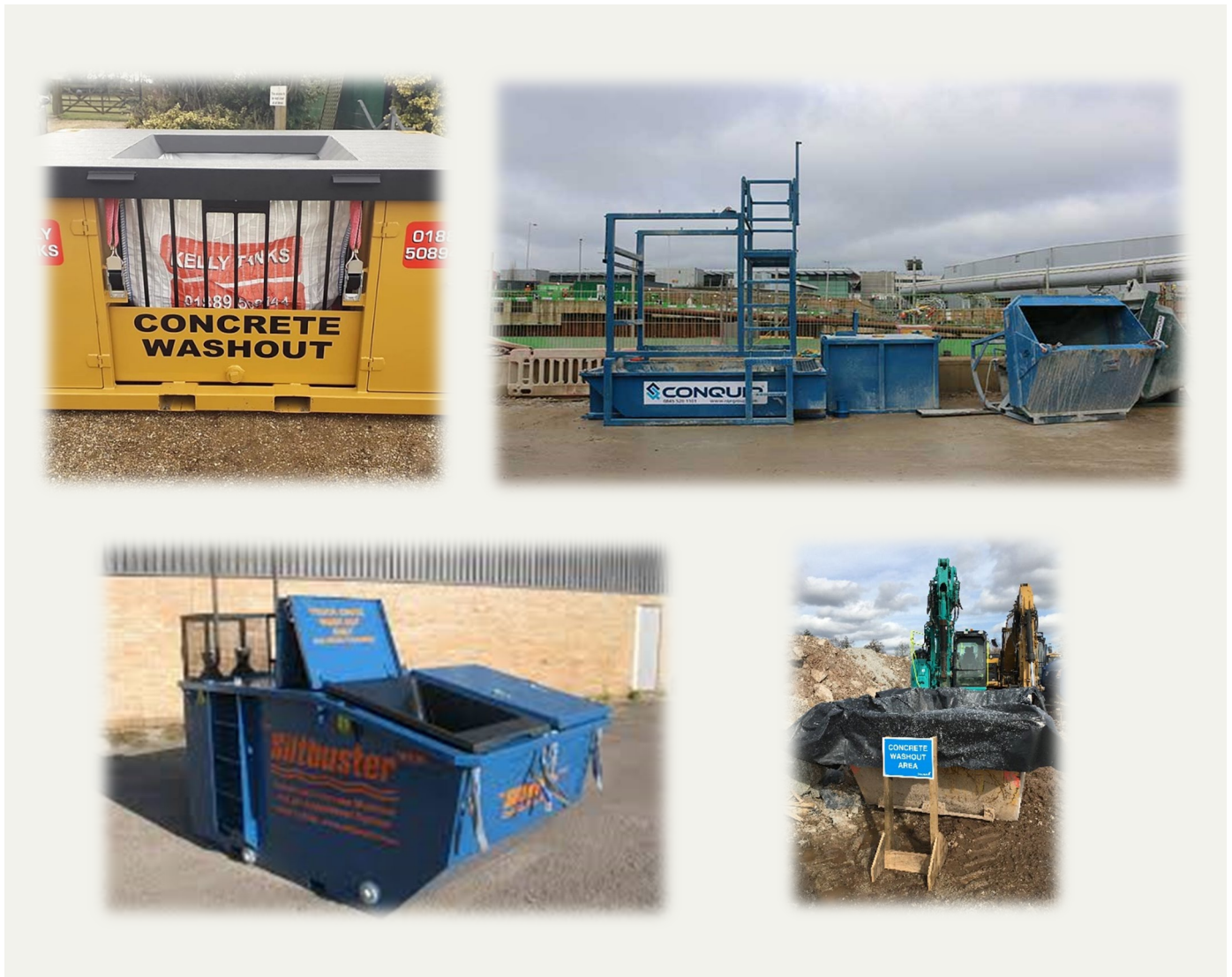
Figure 7 - Examples of Concrete Washout Systems that may be utilised on site
